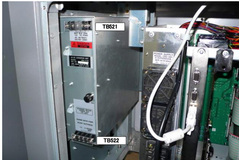
Fig 3-16: Equipment 6 of NBA-5135 (NCD-4990)
