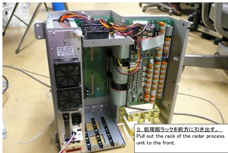
Fig 3-12: Equipment 2 of NBA-5135 (NCD-4990)
